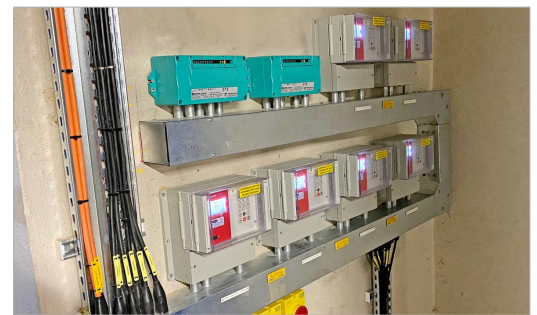
KATflow 150 non-invasive clamp-on flowmeters measuring raw activated sludge at a wastewater treatment plant in South England.
