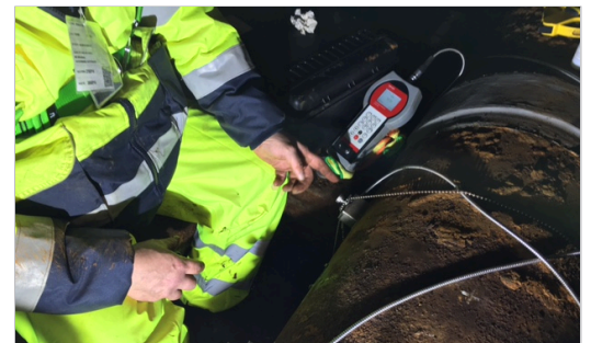
A KATflow 200 portable flowmeter was used to survey the pipe prior to full installation.
